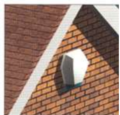
Front active alarm bell box
